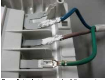
Figure 3: Heat sink paste at L & N connections
